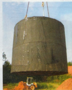
Fig. 1 Installation of the concrete cistern with thermal insulation on its outer cylinder surfaces.
